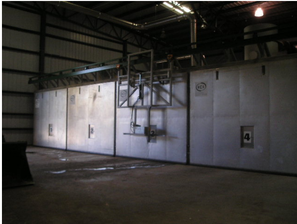
ECS in-vessel compost vessel
